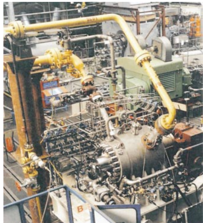
Fig. 10 Photograph of the reinjection compressor
